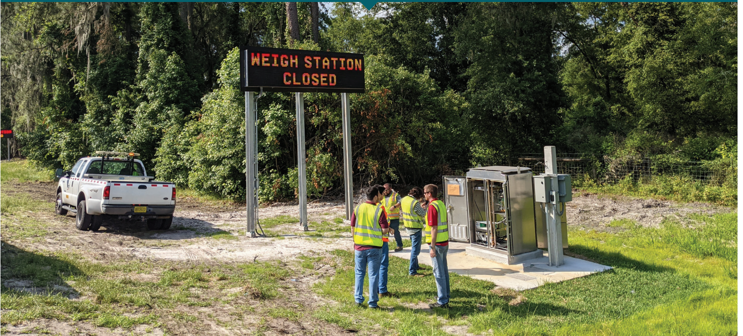
Location: Florida | FDOT MCSAW Fiber Optic and Electronic Trucking Bypass System
